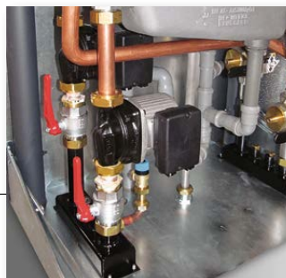
Pumps and gate valves
